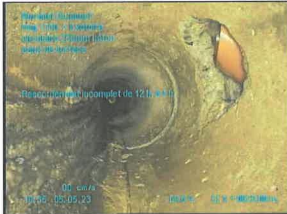
25, 00:09:44, 29.00m Raccordement incomplet de 12 h. à 4 h.
